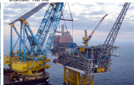
Topside and Decks
